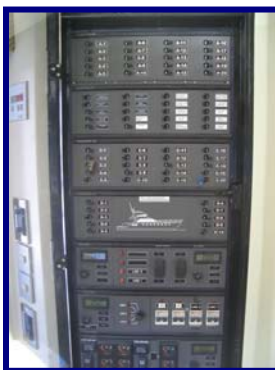
New Electrical Panel
